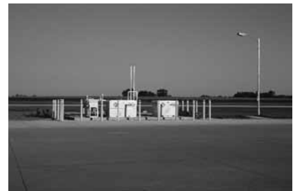
The new fuel system.
